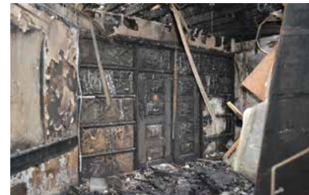
Internal side of fire door after fire
