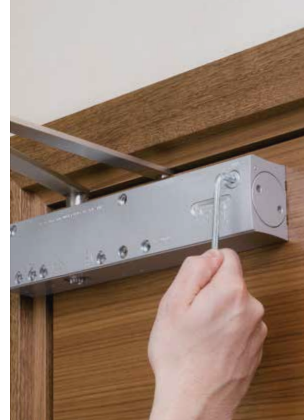
Door closer maintenance
