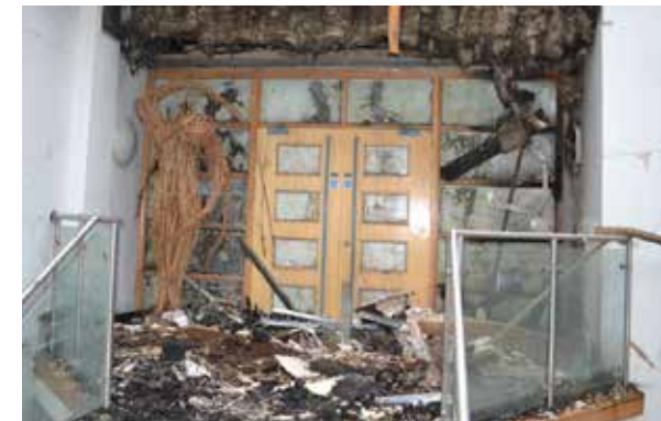
External side of fire door after fire
